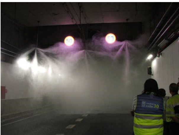
Fig. 1: Activation of a water mist FFFS in a tunnel on the M30 in Madrid (Source: IFAB)
