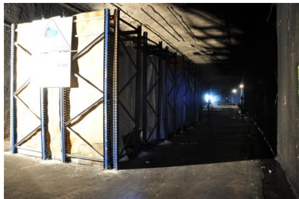
Fig. 35: Typical fire load without chassis to give a larger distance between the fire load and the tunnel roof
