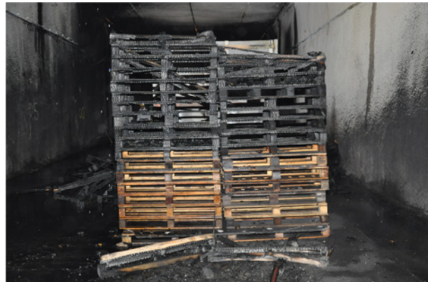
Fig. 16: Spread of fire to a further object at a distance of 5 m during a fire test without FFFS
