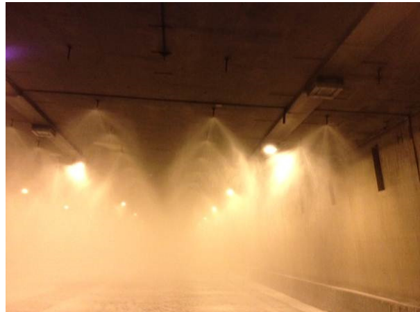
Fig.2: Activation of an FFFS deluge system in Mount Baker Tunnel (I-90) in Seattle (Source: IFAB)
